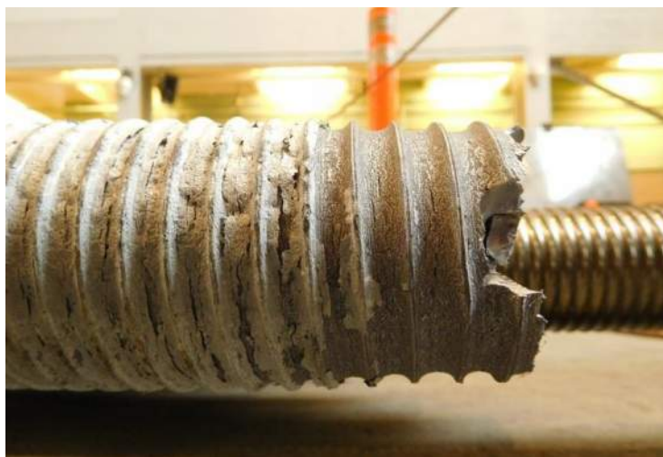
(c) Cracking and flaking of the galvanized coating in the failure region.
