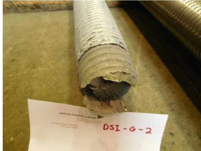
(a) End view showing loss of the galvanized coating.
